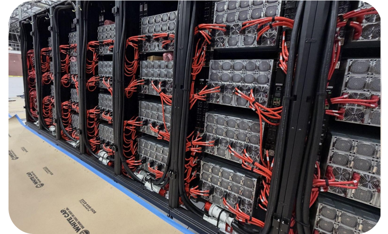
GPU RACKS IN BUILD
